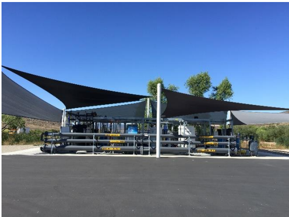
Caption: Advanced Water Purification Demonstration Facility
