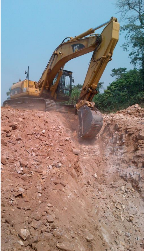
Caption: Hard dig on pipeline installation project requiring a small bucket and heavy breaker
