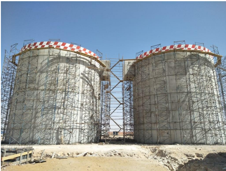
Caption: Laayoune Wastewater Treatment Plant in Construction – Digester Tanks One and Two
