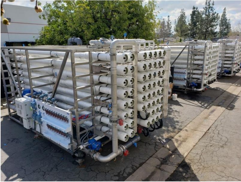
Caption: Biwater Inc's. reverse osmosis trains ready to ship
