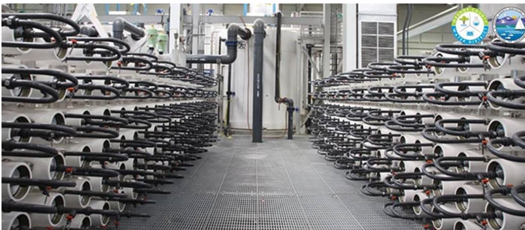
Caption: Orange County's Groundwater Replenishment System, the world's largest facility for indirect potable reuse at 492,000 m 3 /day (130 MGD).
