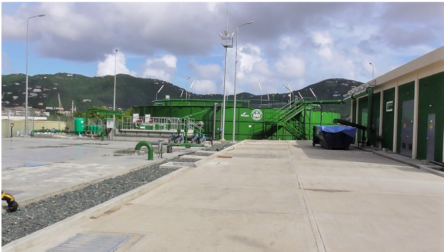
Burt Point package wastewater treatment facility, February 2016
