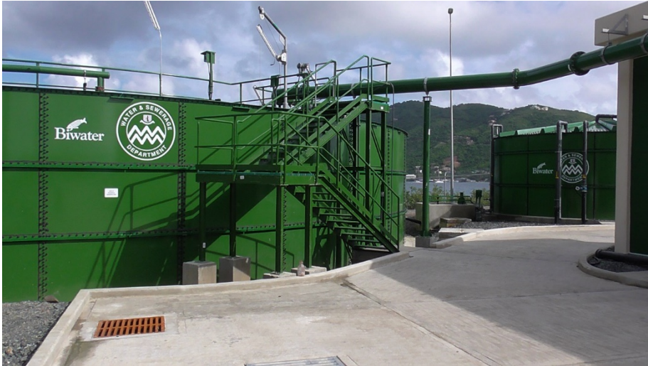
Burt Point package wastewater treatment plant, Bicom Model 3000N, February 2016
