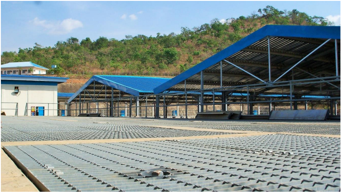
Image taken from the Lower Usuma Dam Water Treatment Plant in Abuja, Nigeria
