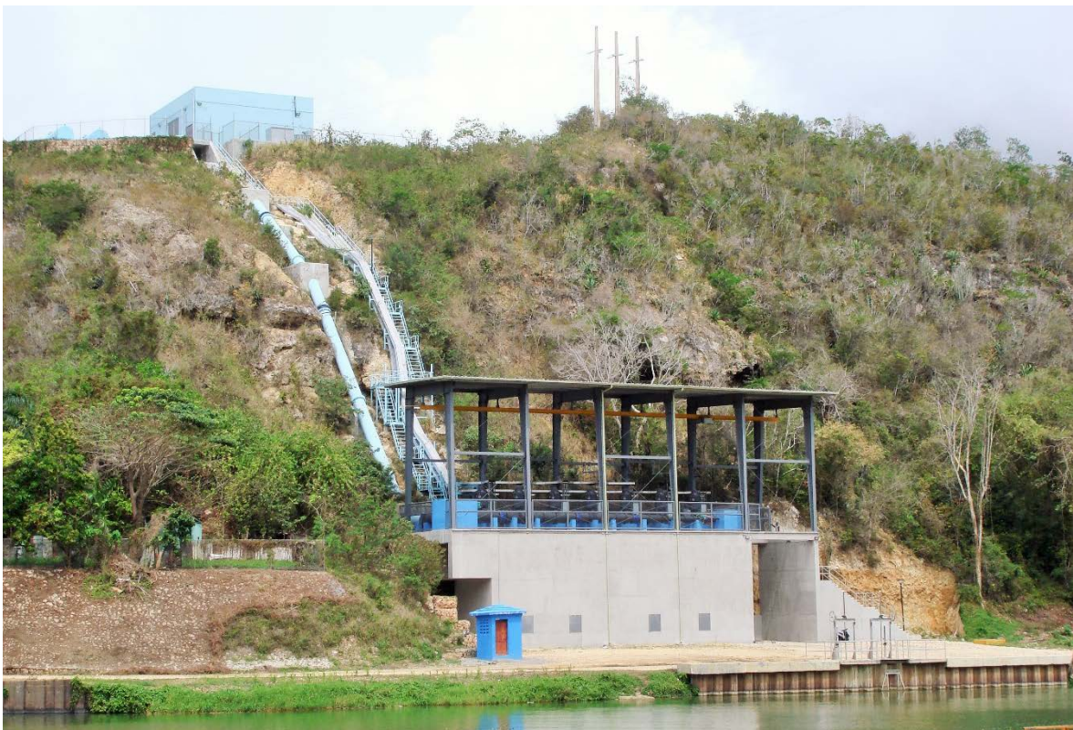
Rio Chavon river intake and pump station for the La Romana Water Treatment Plant in the Dominican Republic
